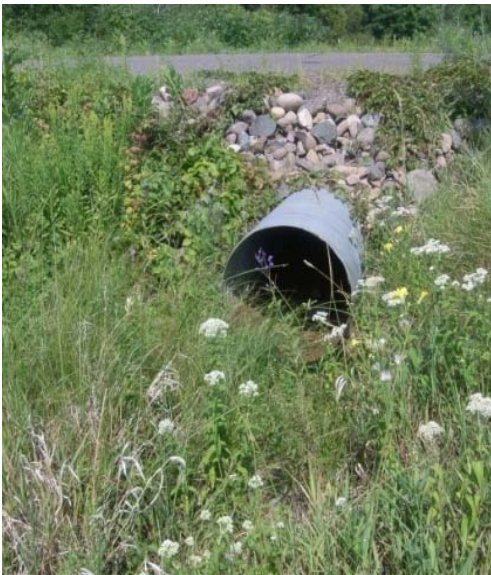
Figure 40. An example of a perched culvert.
